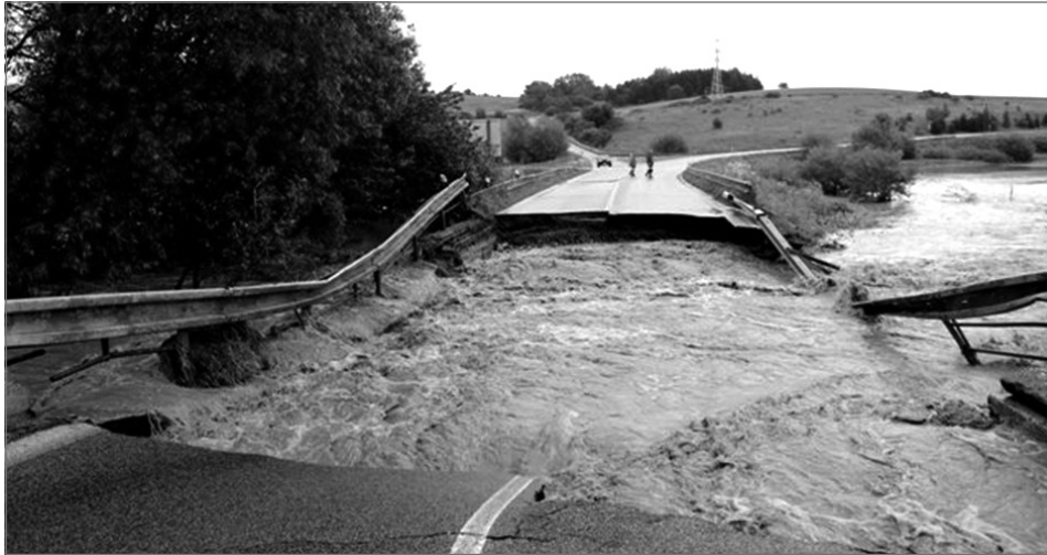
Fig. 14. Torn off part of bridge beyond town Spišská Nová Ves
